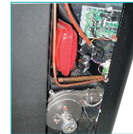
Expansion vessel, flue gas fan
